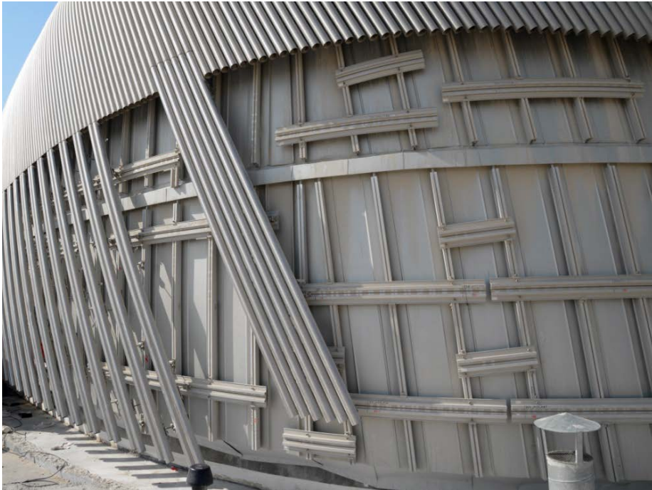
Building the façade with 350km of stainless steel tube bent in three dimensions. ©seele/Michael Vogt
