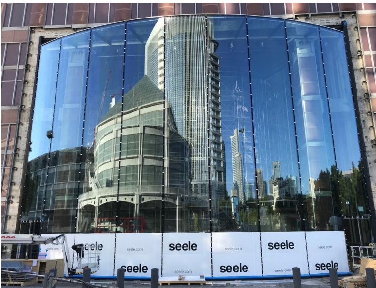
The first façade segment with its nine cold-bent insulating glass units was completed at the end of August. © seele
