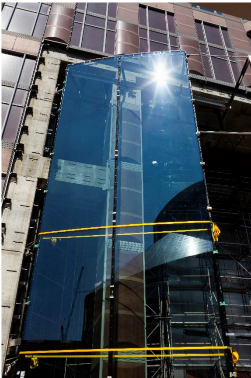
Each façade segment consists of nine cold-bent insulating glass units measuring 17 x 2.8m. © Jessica Schäfer
