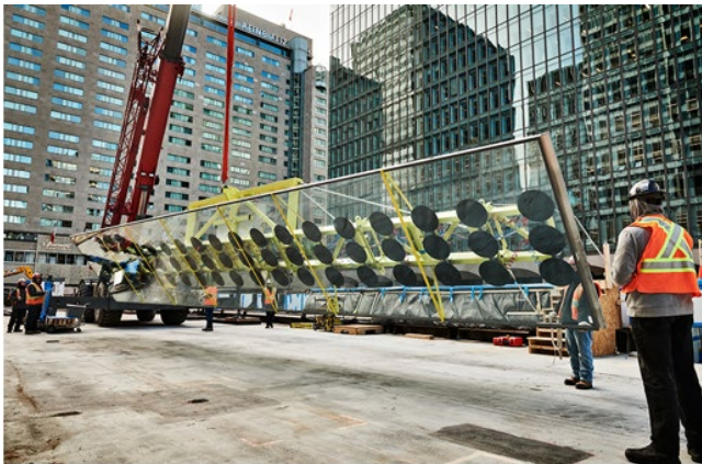
Vacuum lifter raising one of the 15 x 2.5m insulating glass units © seele
