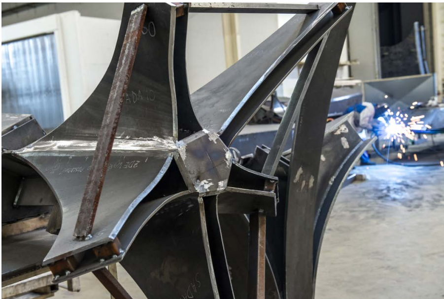
Production of steel tree columns for the project Château Margaux at seele pilsen. ©seele/René Müller
