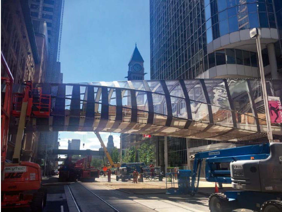
The lifted CF TEC Bridge between Hudson's Bay Shopping Mall and Toronto Eaton Centre (TEC) in Queen Street West in Toronto. ©seele
