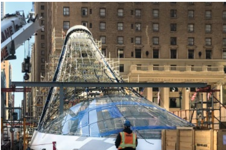
The challenging construction in the heart of Manhattan called for expert coordination of all site works. © seele
