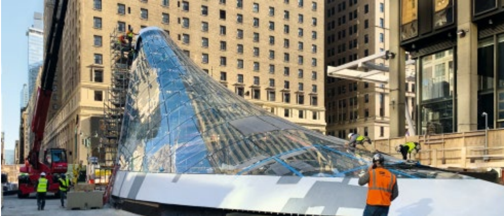
The last pane of glass was installed in November 2020 and the entrance was officially opened for commuters and travellers on December 31, 2020. © seele
