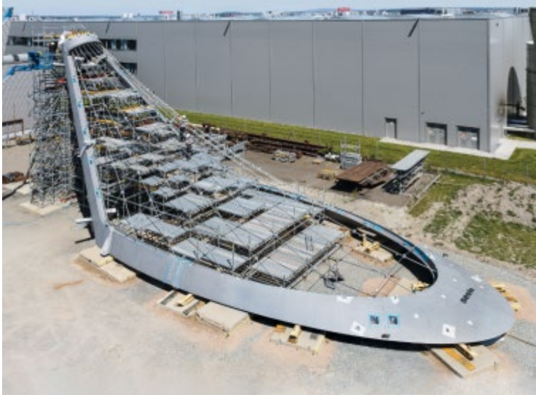
Trial assembly and testing of the steel structure for Penn Station was carried out at seele pilsen in the Czech Republic before being shipped to New York. © seele
